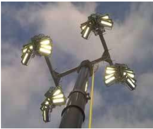
HH SHEIK JASSIM PALACE LIGHT INSTALLATION
