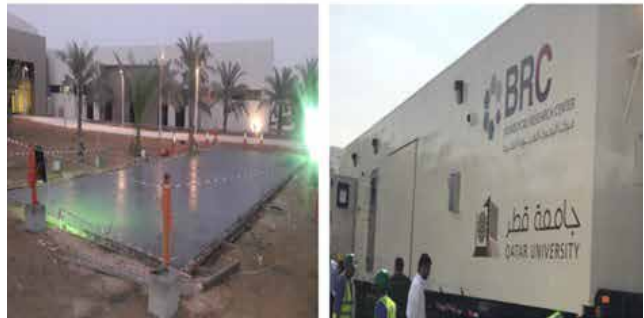
MEP Works to connect the BSL-3 Mobile trailer Laboratory with existing facilities at H10 building in Qatar University.
